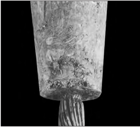
Typical example of the swelling of stainless steel rope due to crevice corrosion
